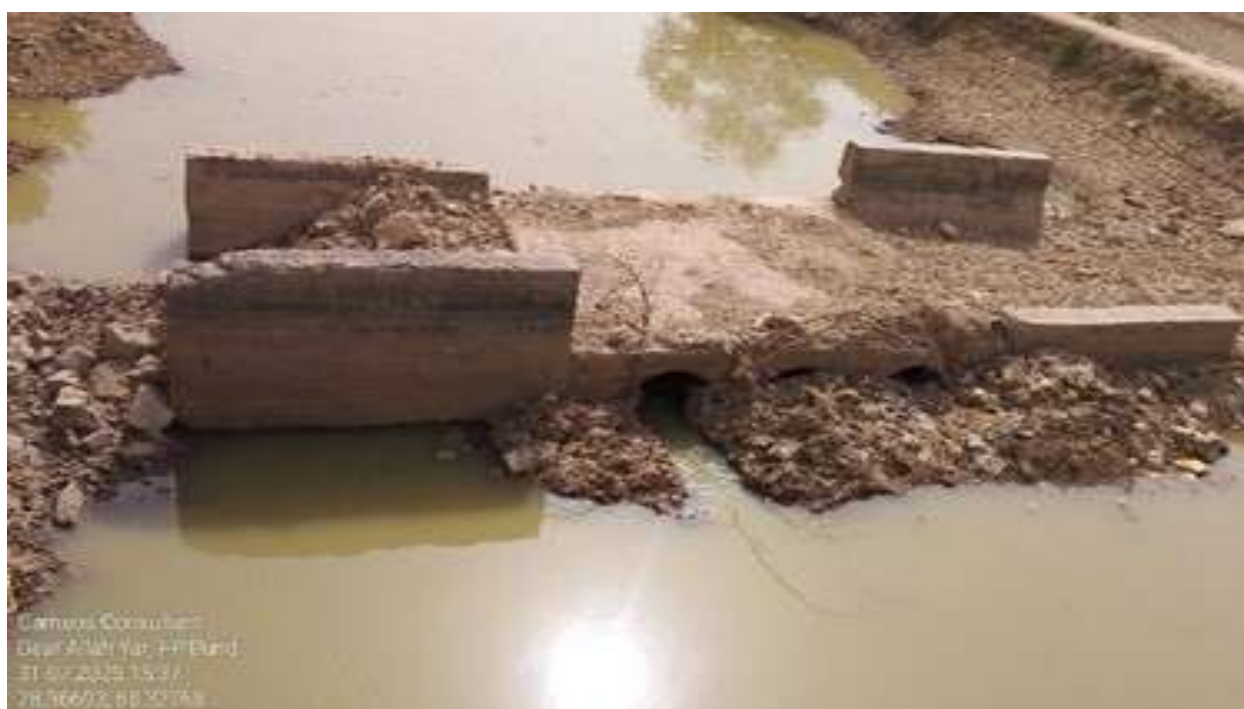
Figure -1-4: Photographs of damaged Super Passages
