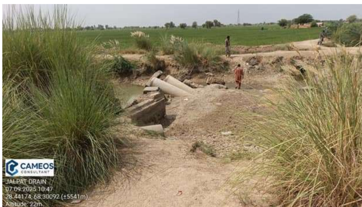
Figure-1-4: Photographs of damaged Flood Protection Bund
