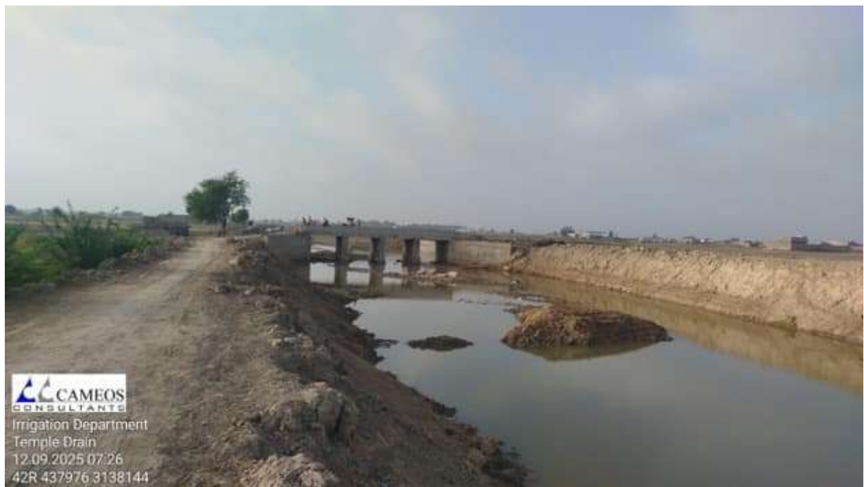
Figure-3-2: Alluvial/riverbed deposits along the washed-out bund.
