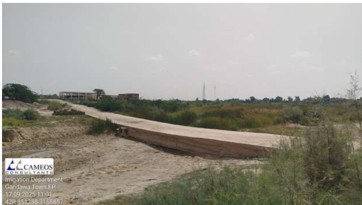
Figure -1-4: Photographs of damaged Gandava FPB
