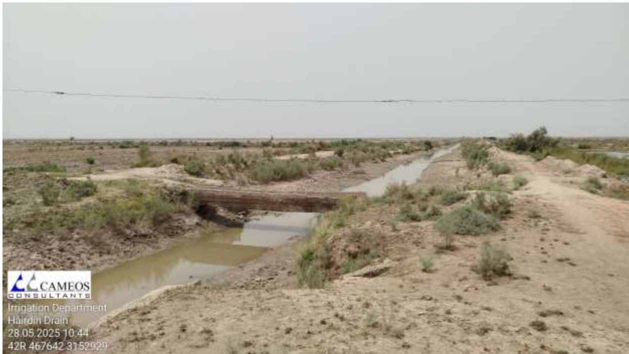
Figure-3-2: Alluvial deposits along the washed-out bund.
