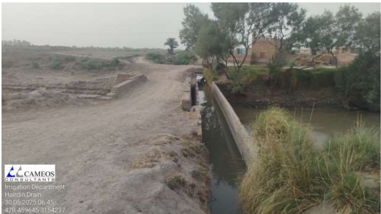
Figure-1-3: Photographs of damaged Zain ul Abideen Flood Protection Bund
