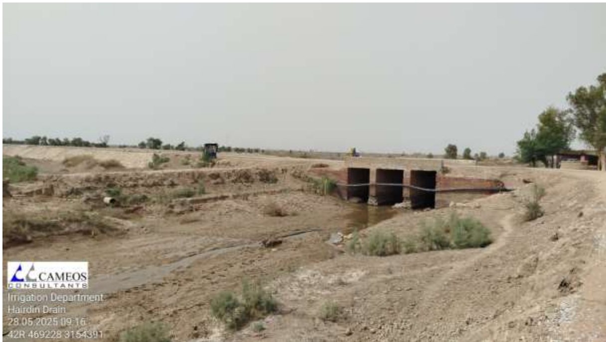
Figure 1-3: Photographs of damaged Hairdin Main Drain
