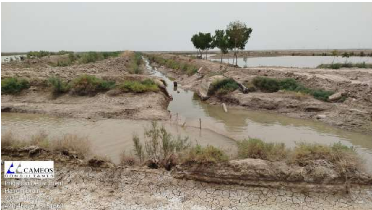
Figure 1-4: Photographs of damaged Hairdin Main Drain
