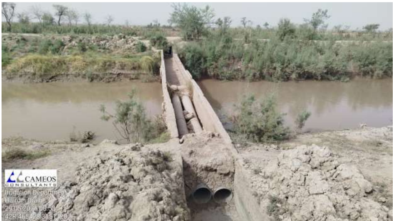
Figure 3-3: Alluvial/riverbed deposits along the washed-out bund.
