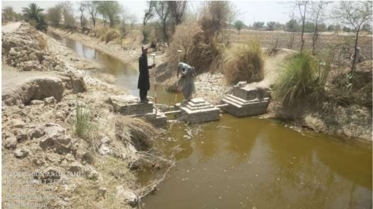
Figure-3-2: Alluvial/riverbed deposits along the washed-out bund.
