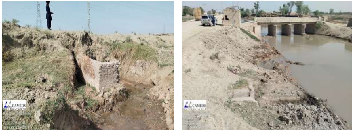
Figure-1-3: Photographs of damaged structure of Uch Canal
