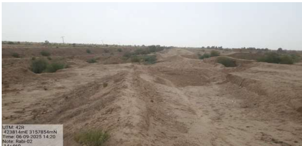
Figure-3.2: Alluvial deposits along the damaged embankment.
