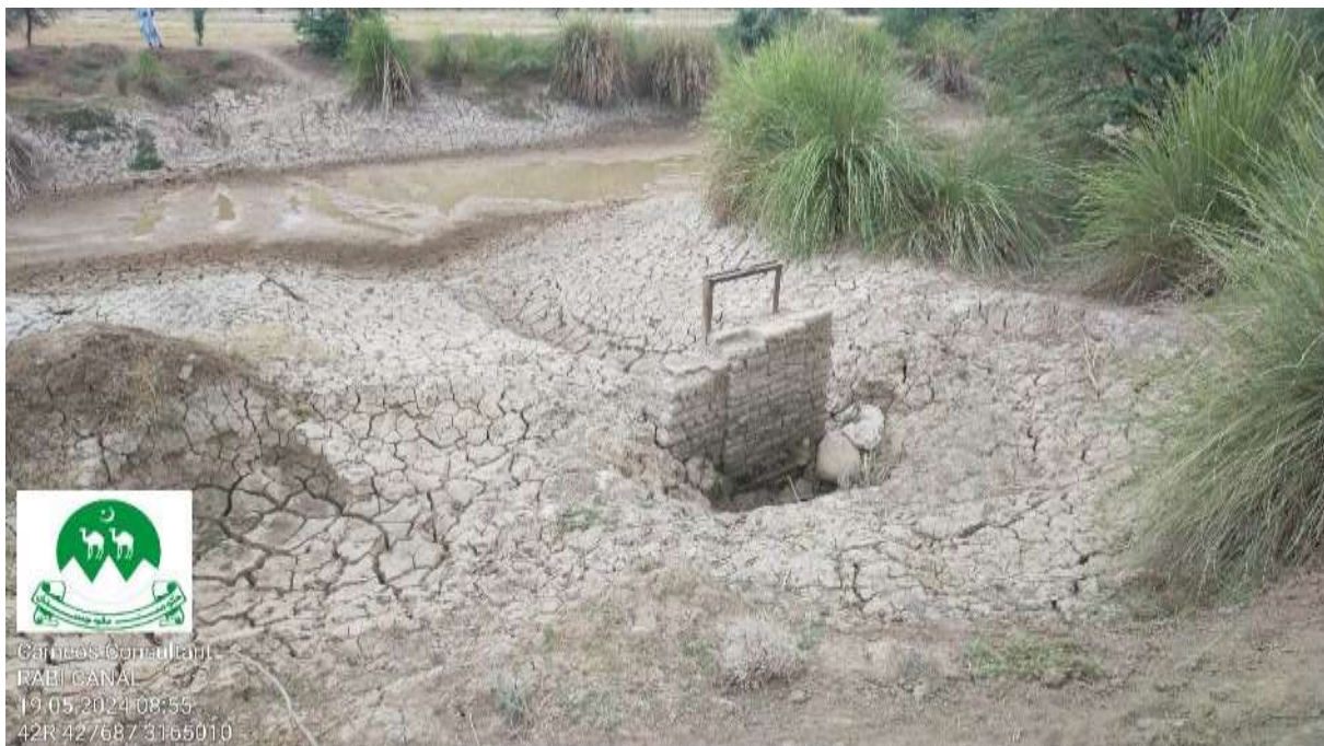
Figure-2: Photographs of damaged Rabi Canal Flood Protection Embankment
