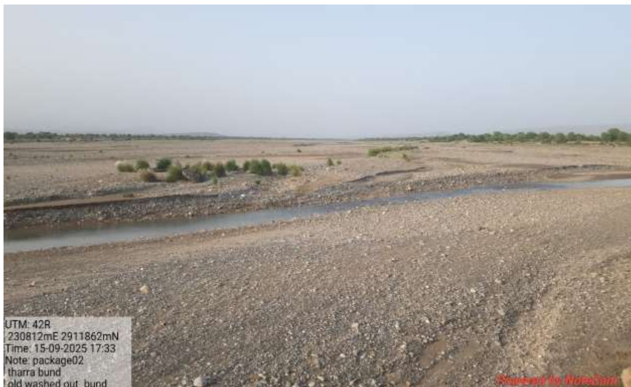
Figure-3-2: Alluvial/riverbed deposits along the washed-out bund.
