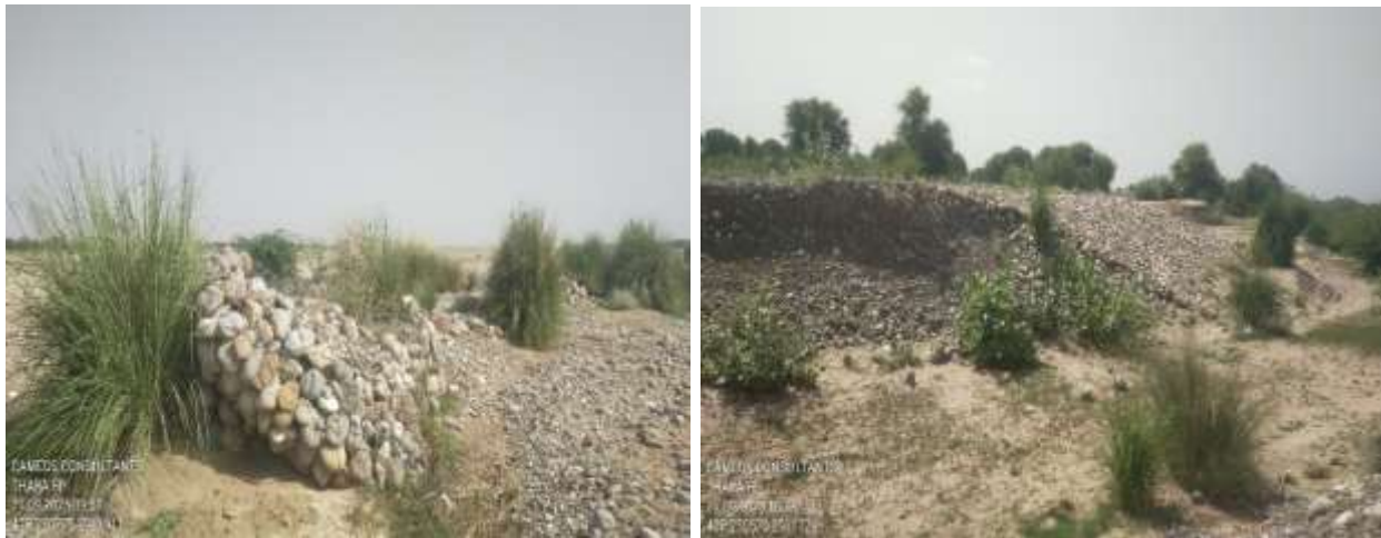
Figure-1-3: Photographs of damaged Thrara Flood Protection Bund
