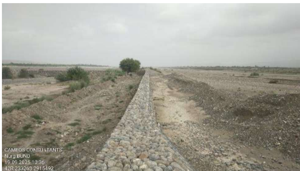
Figure -1-4: Photographs of damaged Faizo & Shurli Bund
